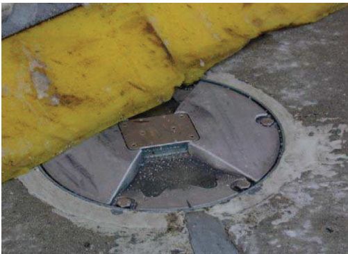
Figure 32: Fig. 2 — Snowplow blade with wear and steps between segments
